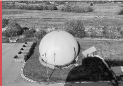
Methane storage tank
